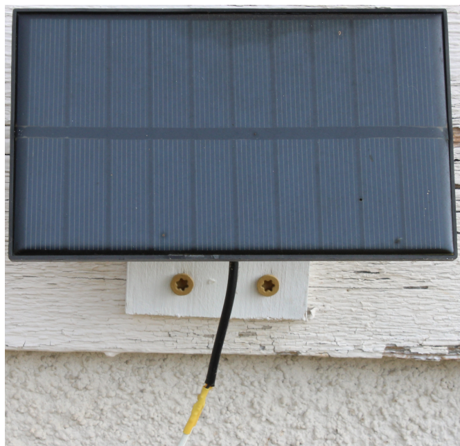
Separated solar cell (over the patio roof)
