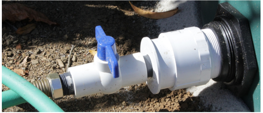
Drain outlet connected to shut-off valve & flexible garden hose
