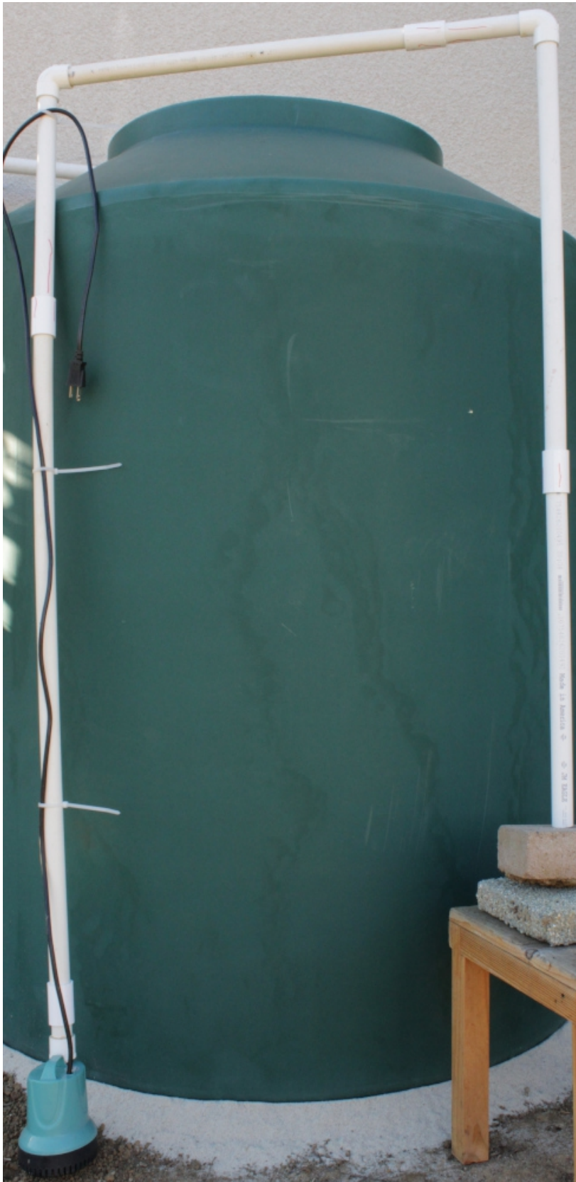
Submersible water pump, PVC pipe & power code routing
