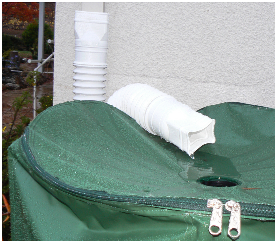
Flexible Downspout Extension to Tank Inlet
