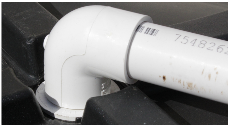
Pipe connection of overflowed rain water inlet (550 gallon rain water tank)
