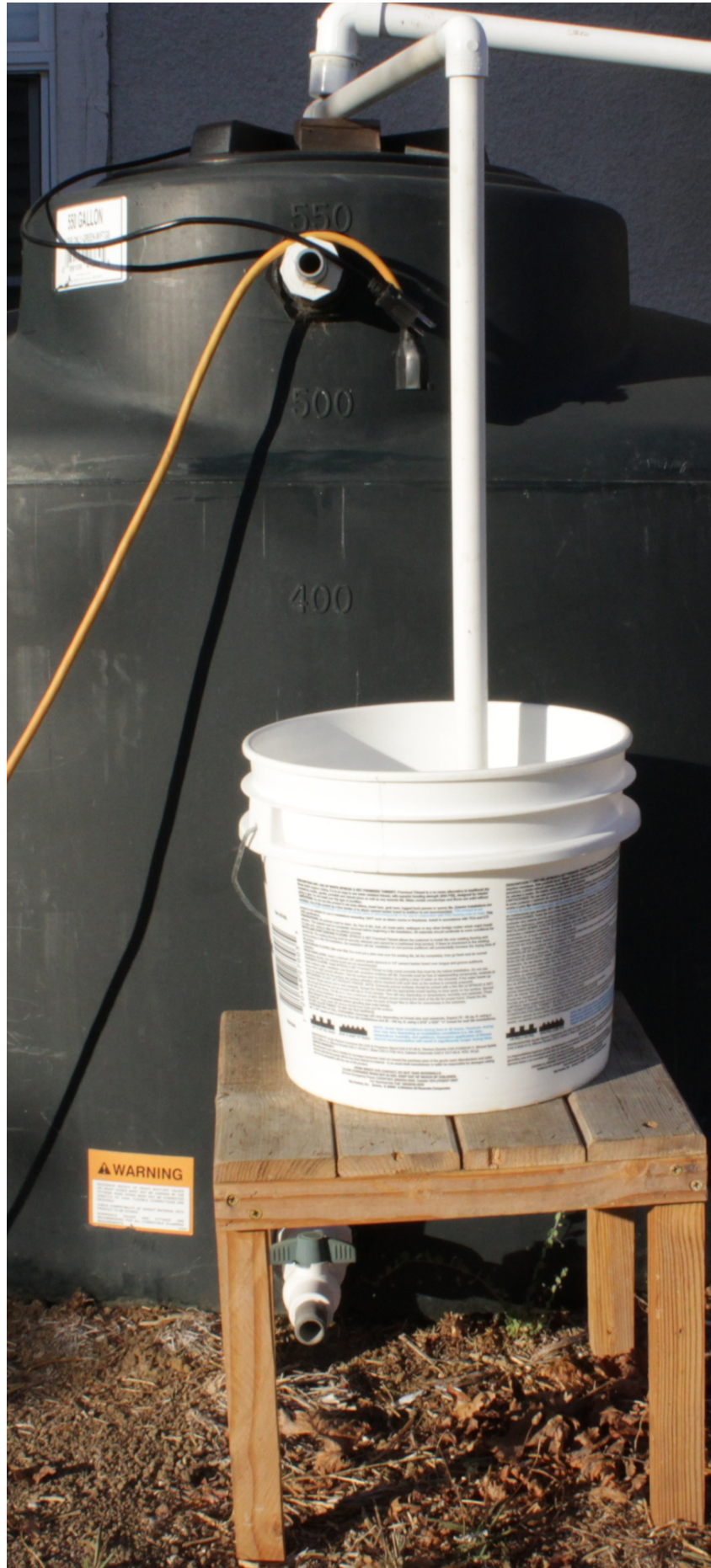
Ready to pump water in 550 gallon rain water tank shrinking the PVC pipe length
