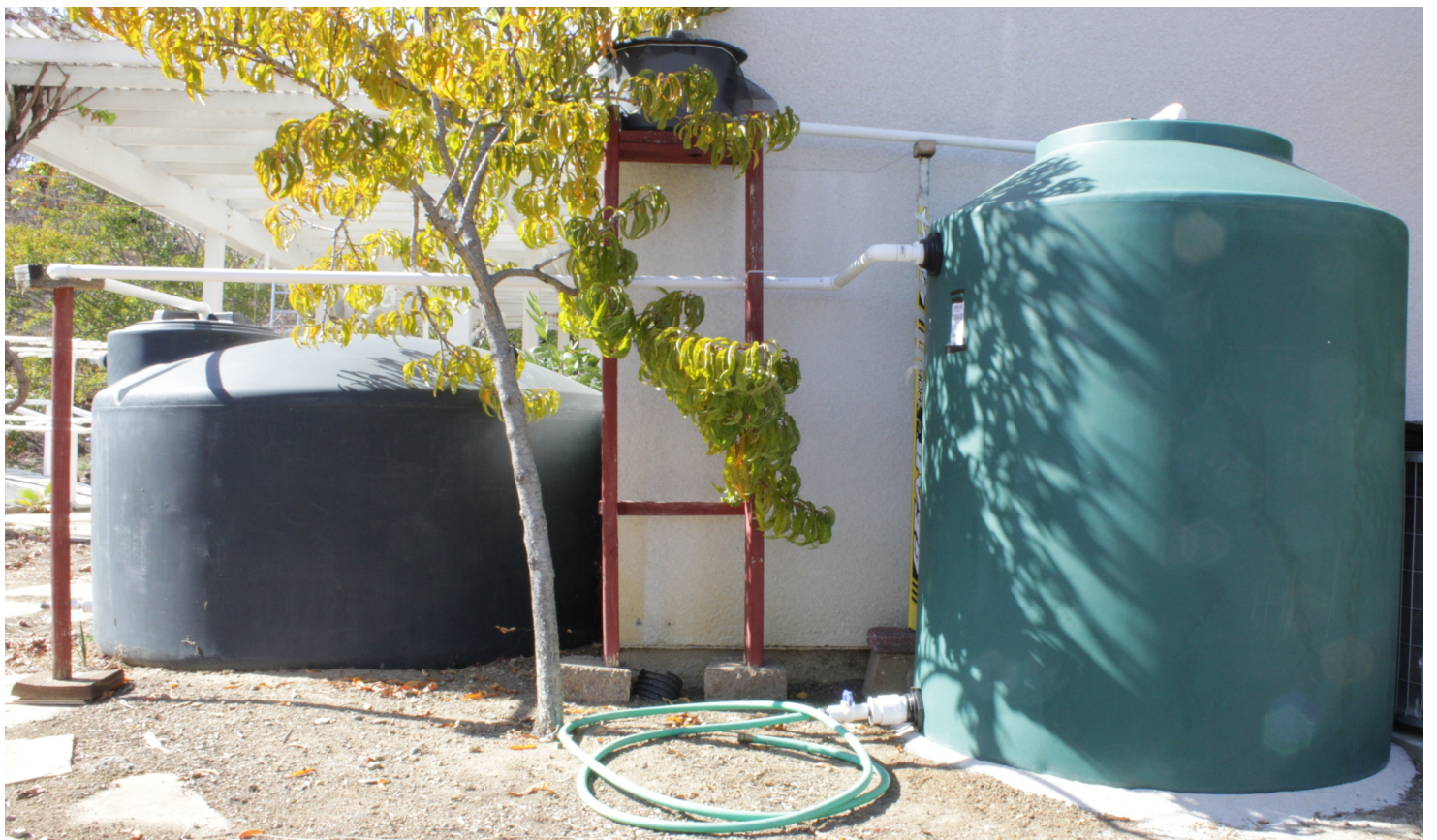
Water pipe connection of 550 gallon rain water tank (Left) and 300 gallon rain water tank (Right)
