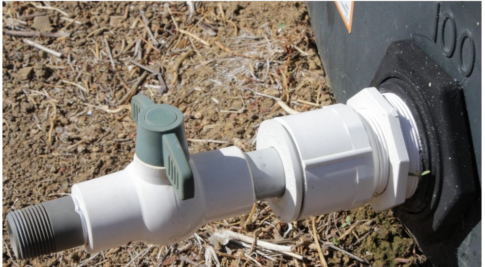
Drain outlet connected to shut-off valve & flexible garden hose nipple
