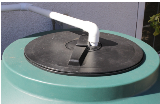
Rain water inlet pipe connection
