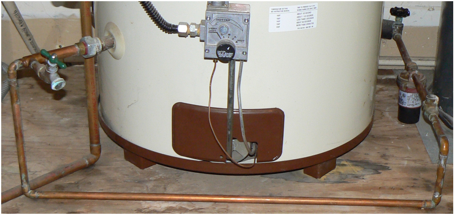
Copper Pipe Routing for Hot Water Recirculation with Circulation Pump (at center right)
