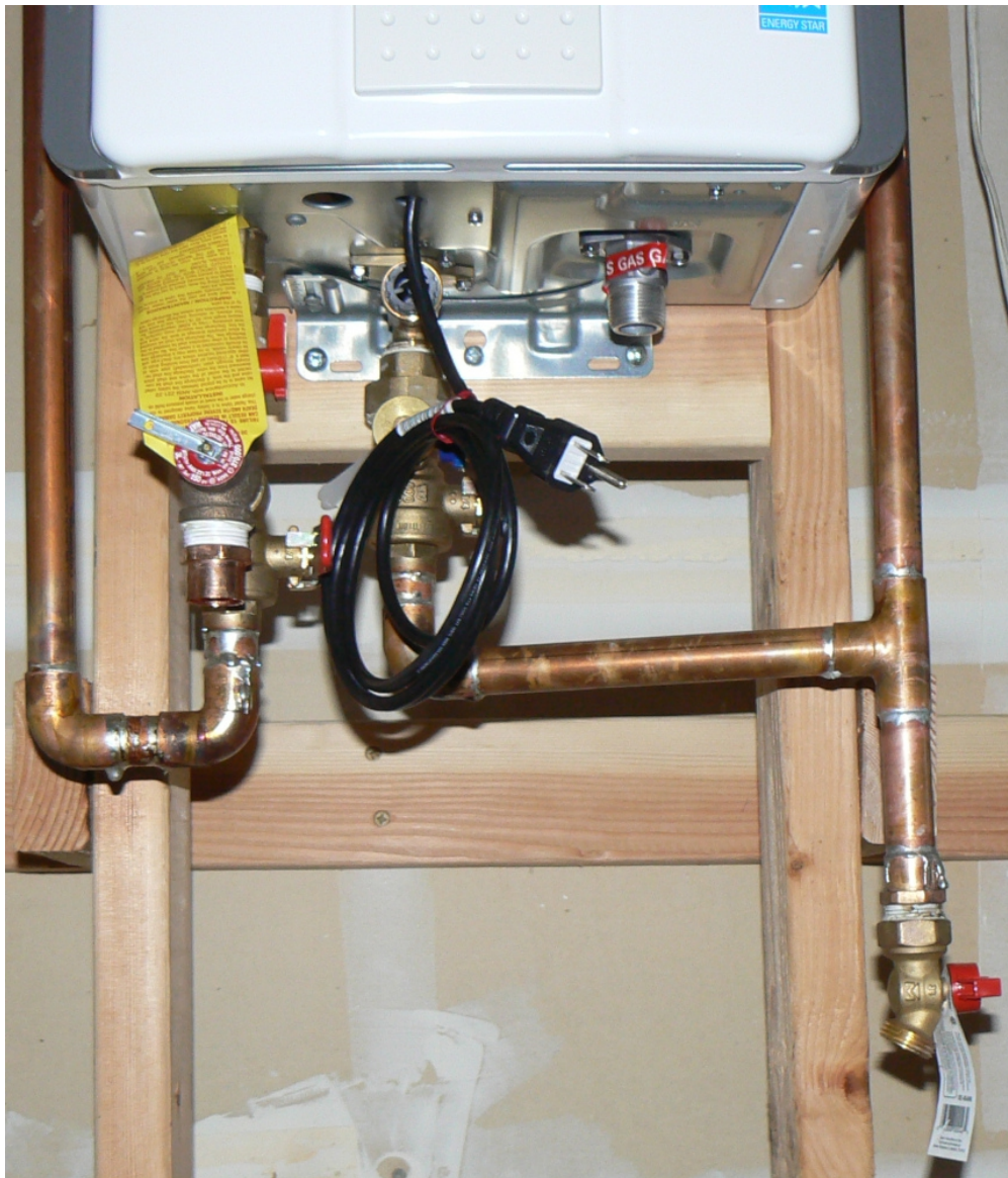
Connection at Bottom with Pressure Release Valve & Cleaning Valves,,,
