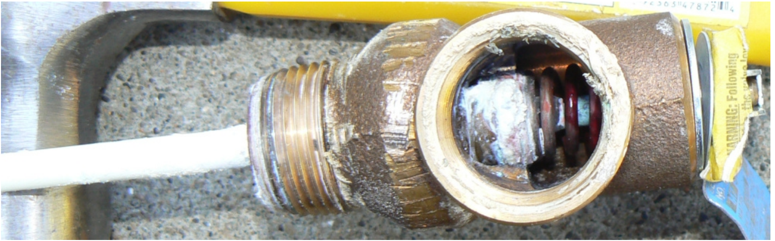
Pressure Release Valve
