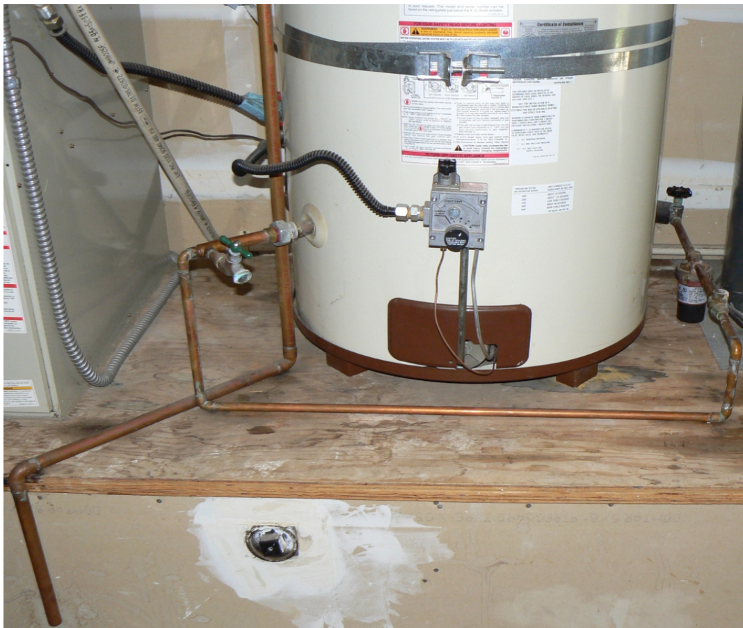
74 Gallon A.O.Smith Water Heater to be Replaced by Tankless Water Heater (Rinnai OEM)
