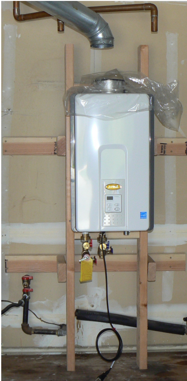
Tankless Water Heater Attached to Wall
