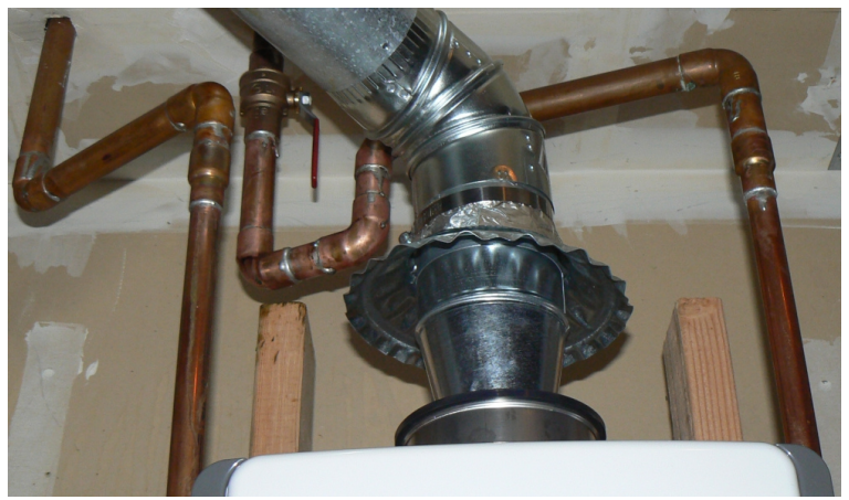
Chimney with Cap Attached
