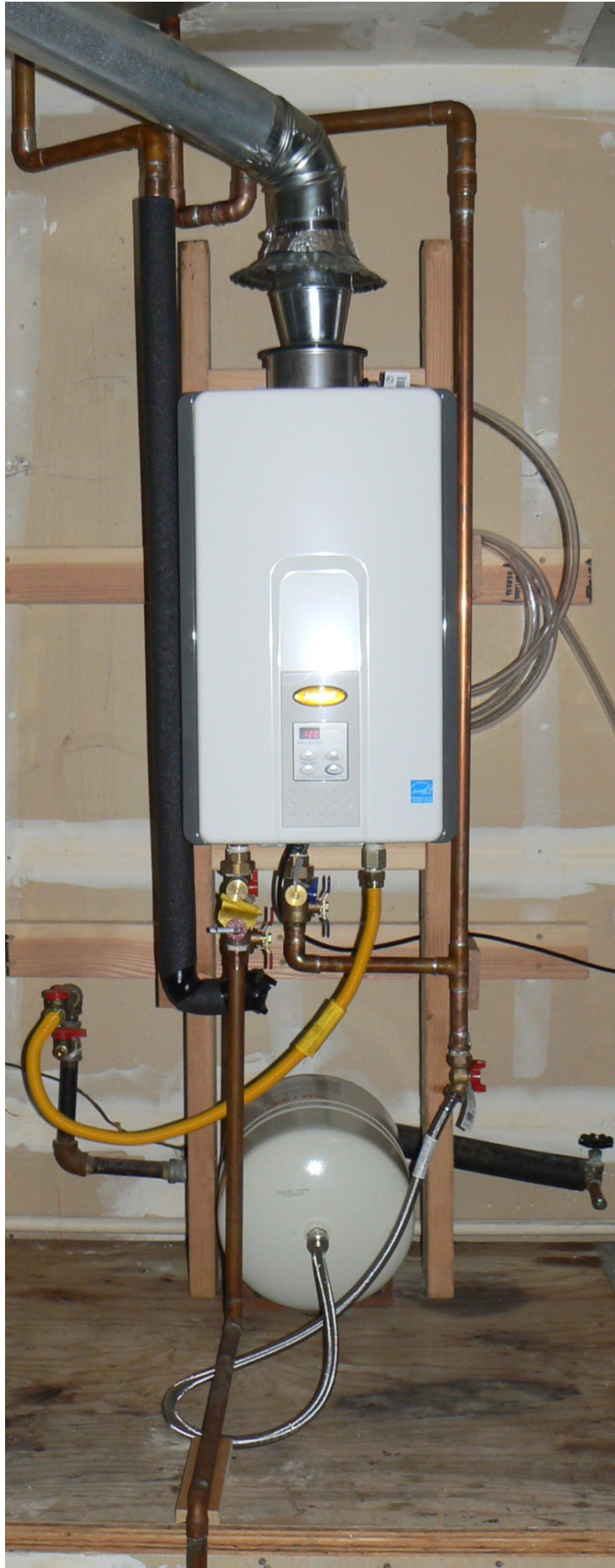
Tankless Water Heater (Rinnai OEM) Replaced with a Thermal Expansion Tank below
