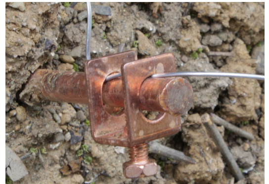
Ground wire connected to earth rod
