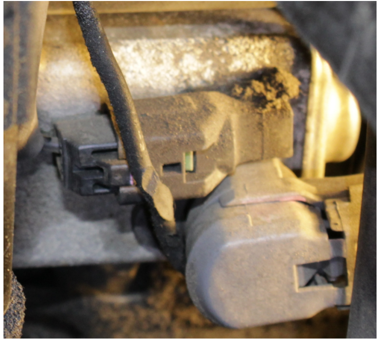
Power & control wire connected
